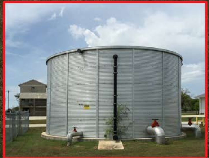
Two 100,000 gallon Pioneer fire tanks at the First Responders Academy in San Antonio, Texas
